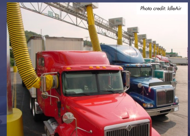
Electrified Parking Spaces offer idle-free heating, ventilating, and air conditioning as well as electric power for appliances.
